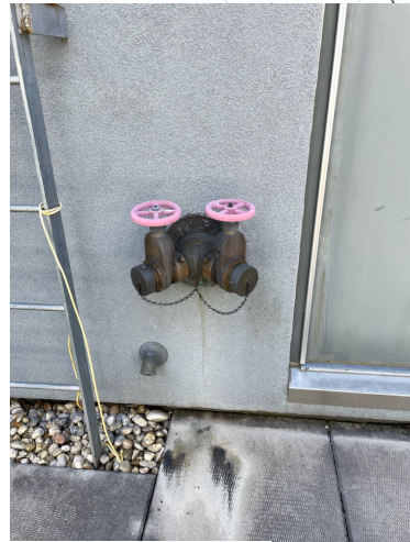
FD Water Connection
