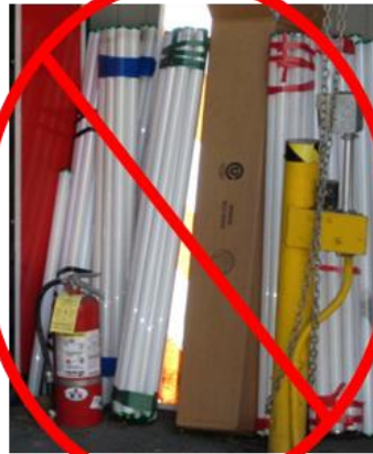
Figure 2. Improper Storage. Bundled lamps stored loosely, leaning upright or slanted against walls with incompatible equipment, risks breakage and penalties.
